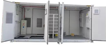
1075KW HH ESS
